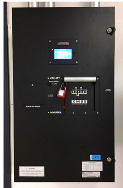
Figure 12: 100A Smart Bypass, Armed for Auto Transfer with Handle Lockout Installed (wall mounted)
