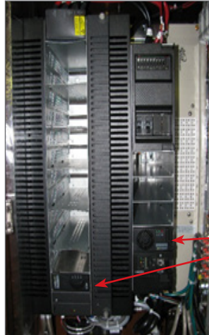
Rectifier and converter modules installed in slot #1 of respective shelves.
